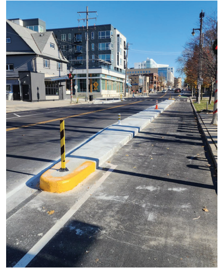
Pinned-on concrete island on southside of the street creating protected bike lane
