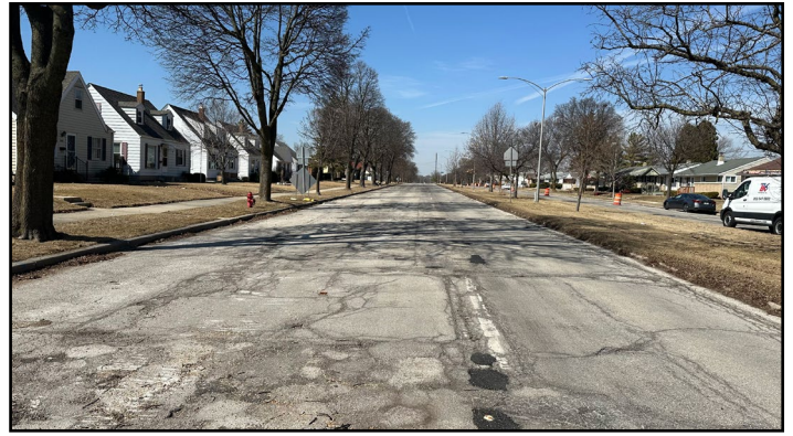
Pre-reconstruction roadway conditions | March 2025
