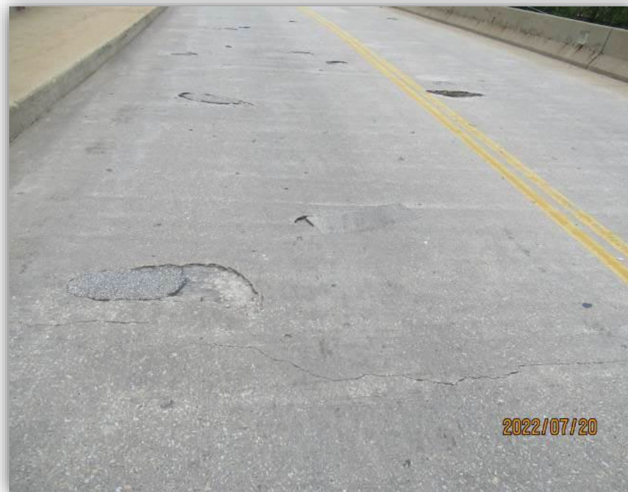
Spalls throughout the top of deck.
