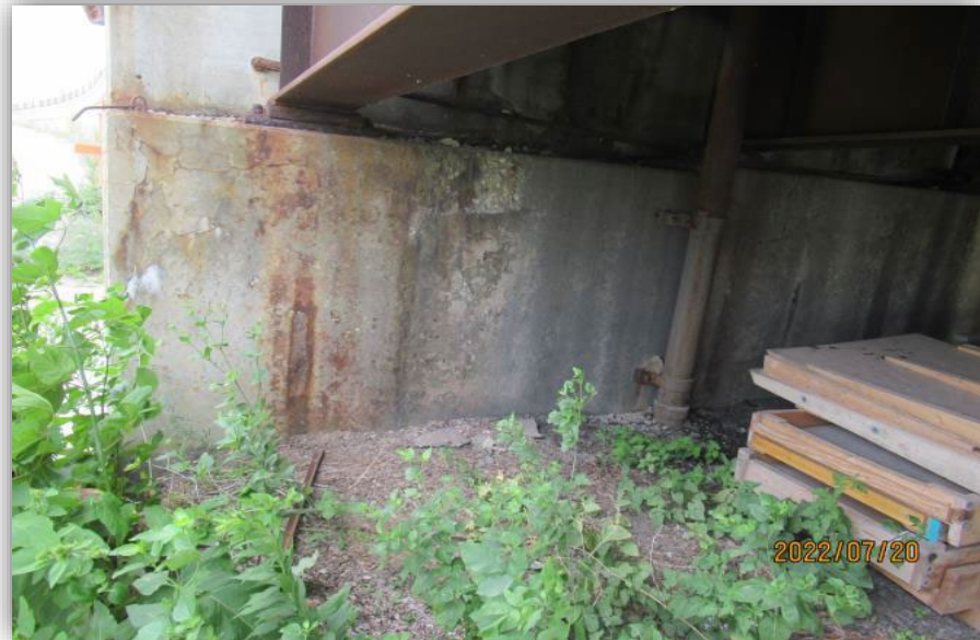
Spall with exposed rebar at the beam seat of girder at south abutment.
