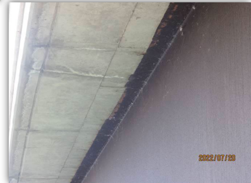
Multiple transverse cracks underside of deck soffit.
