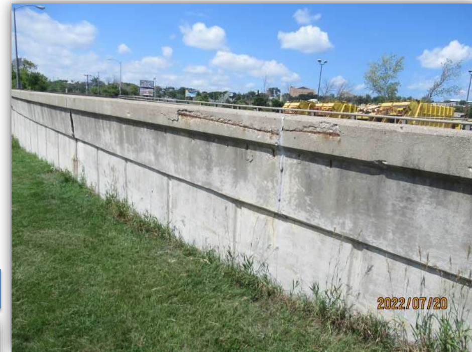
Spalls with exposed rebar along concrete railing at west face of the cellular abutment
